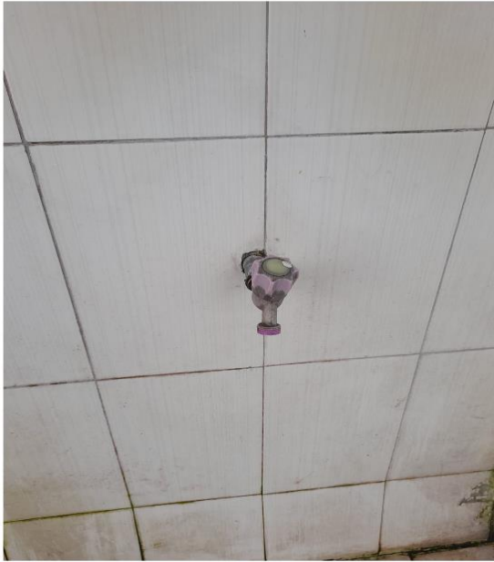
d. Kran mushola bocor
